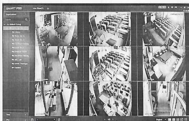
Grid of CCTV Camera
